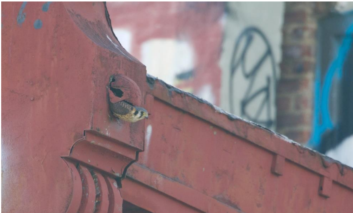
Kestrel nesting in rusted-out building cornice in New York City (photo by Jean Shum)
